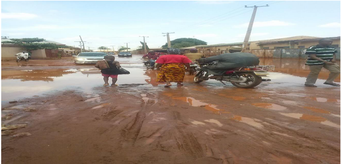
Plate 5: Road Constructed without Drainage (Site 1)
