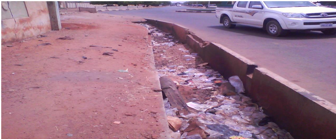
Plate 1: Kerbs Falling into Drainage (Site 2)
