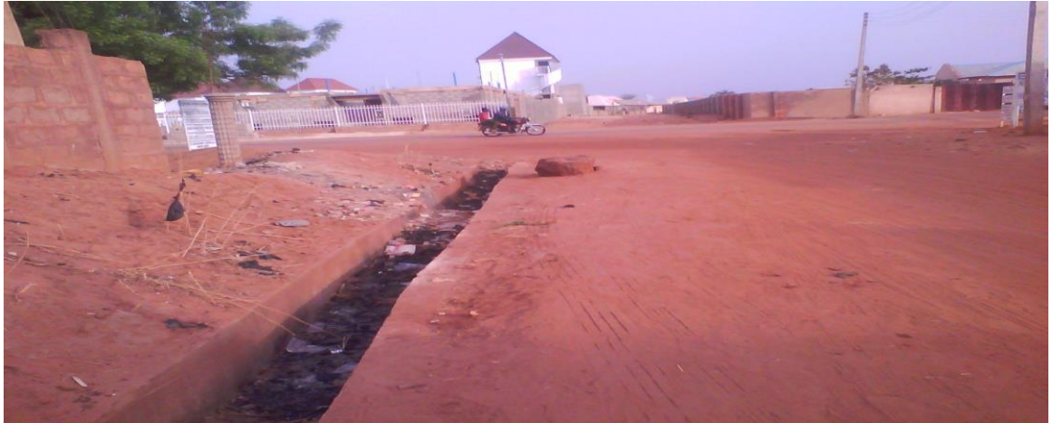
Plate 2: Drainage without Outlet (Site 3)
