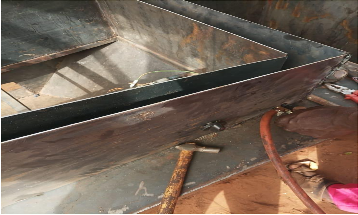
Plate 6: Positioning of a gas cylinder for generating gas to the burner (ignitor) in progress
