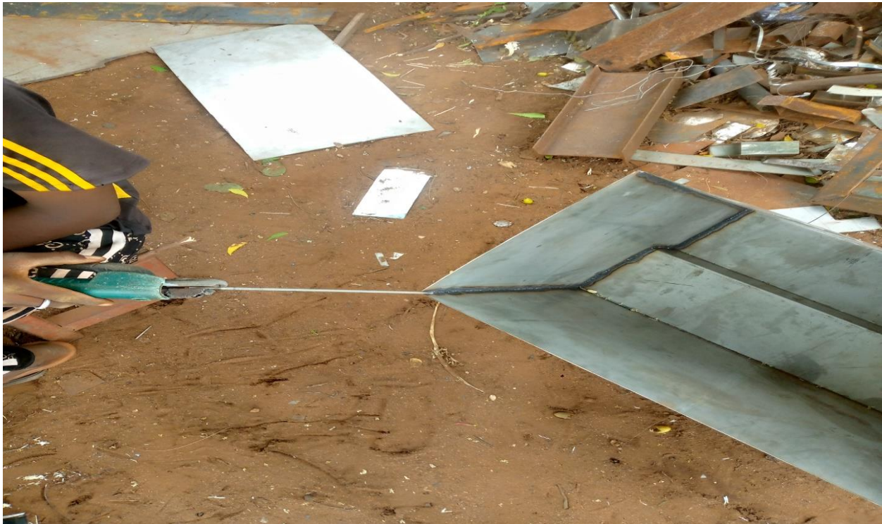
Plate1: The welding connection in stainless steel use in the Fabrication Work after the parameter was designed.
