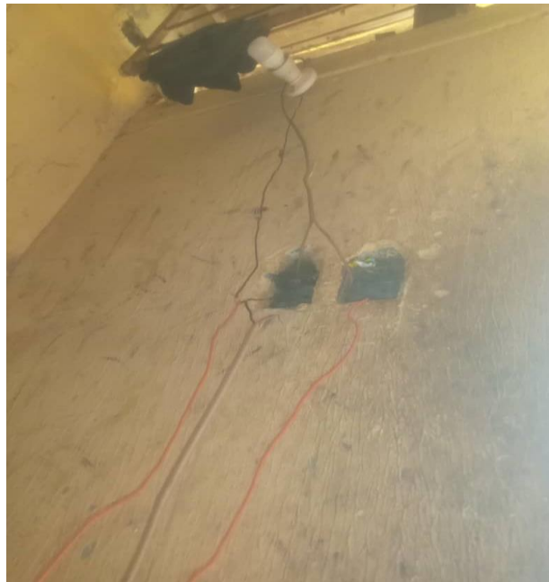
Figure 8. Single core cabled used for surface wiring .instead of twin PVC Cable.
