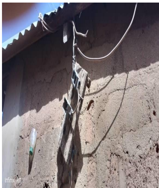
Figure 12. Consumer terminals suspended on Meter board
