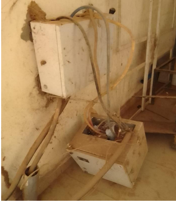
Figure 16. Dismantled 415volt gear switch resting on Floor while in use.
