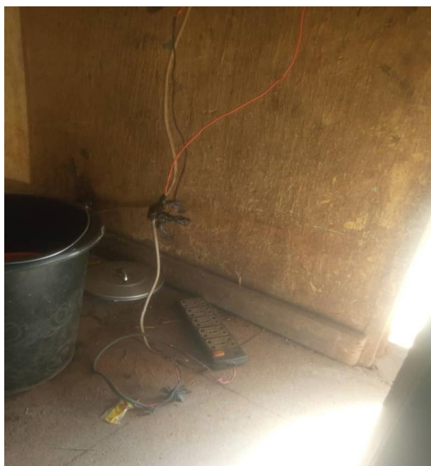
Figure 11. Exposed 1mm 2 single core cable used to on Power heating devices.
