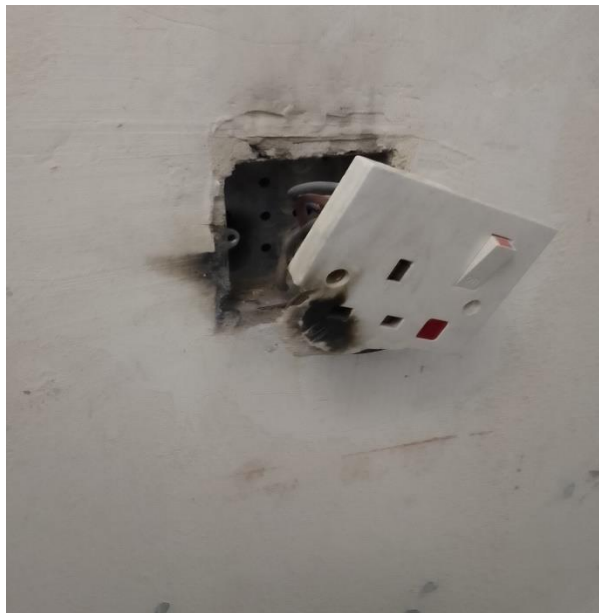
Figure 14. Short circuit due to improper termination.
