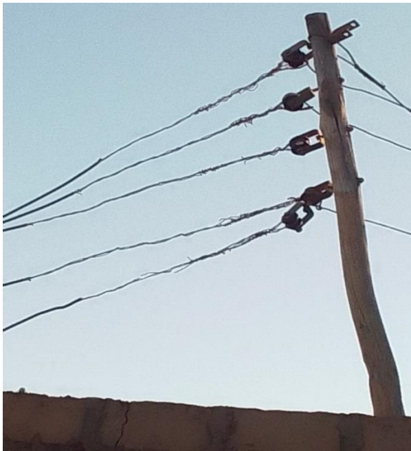
Figure 7. Undersize 415 volt Service cable and Wooden pole.
