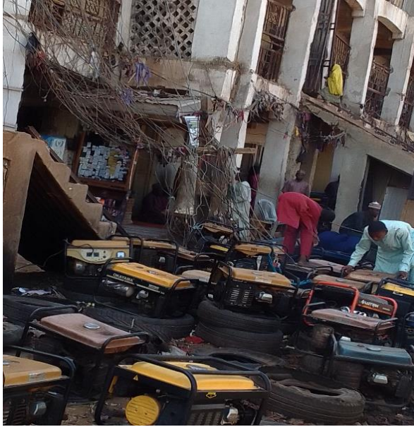
Figure 1. Electric generators under sun supplying Cables exposed to Shops in a market
