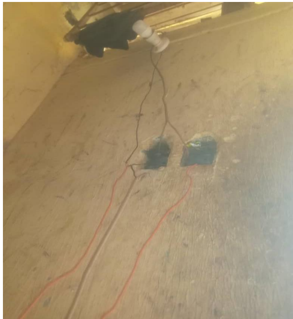
Figure 13.Exposed 1mm 2 cable supplying both supplying Socket and lightings.
