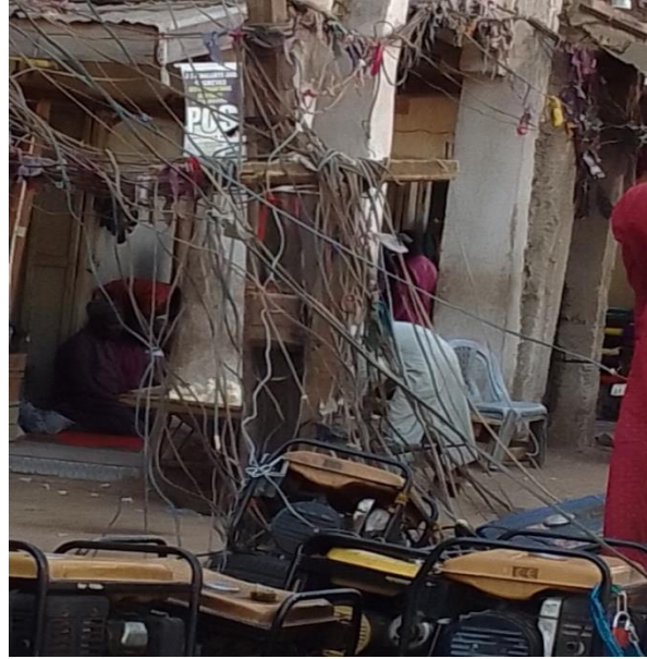
Figure 2. Improperly arrange PVC to sun.
