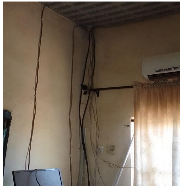
Figure 15. Improperly installed cables
