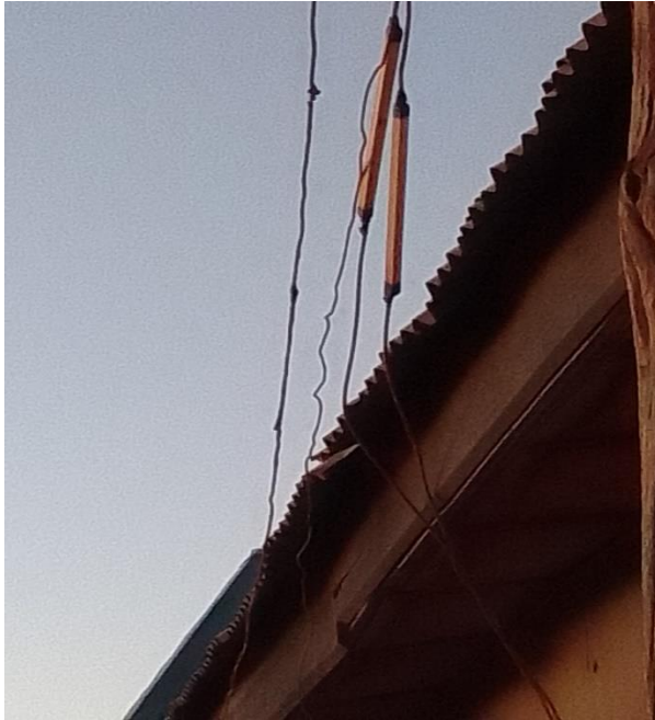
Figure 5. 415volt service cable in contact roofing with zinc
