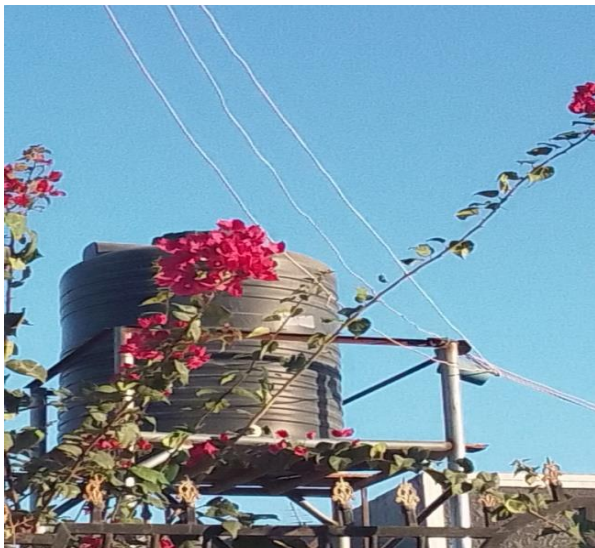
Figure 3. Low tension service cables supported and nest directly by galvanized iron overhead tank stand.
